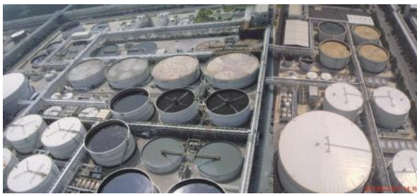
Wastewater treatment plant (before improvement)
